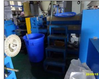
Photo of non-conformity 7.17 no no handrail for ladder.JPG
