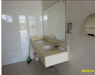
Photo of non-conformity 7.22 no soap in the basin.JPG
