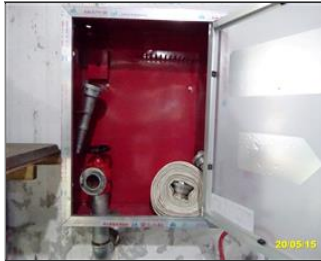
Photo of fire safety equipment fire hydrant.JPG
