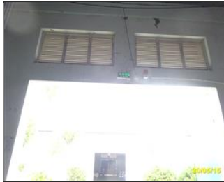
Photo of fire safety equipment emergency light exit sign fire alarm.JPG
