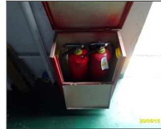
Photo of fire safety equipment fire extinguisher.JPG
